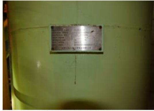
煙氣冷卻塔水槽
