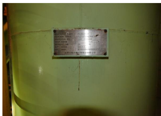
煙氣冷卻塔水槽
